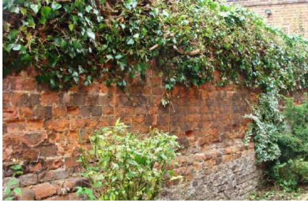
Picture 38. Important wall to south of Almshouses in need of repair.
