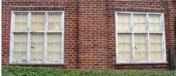
Picture 29. Early windows to Nisa Local Store and PO worthy of retention and in need of refurbishment.
