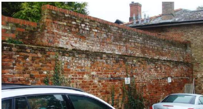
Picture 39. Good quality tall brick wall to rear and north of Town Council offices. Suggest removal of ivy whilst young and easy to achieve.
