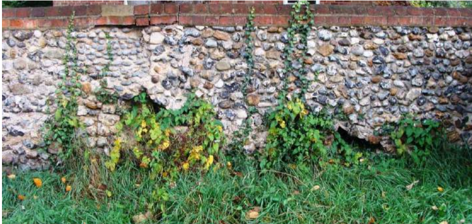
Picture 45. Boundary wall to New Cottage, The Causeway in need of repair and removal of vegetation.
