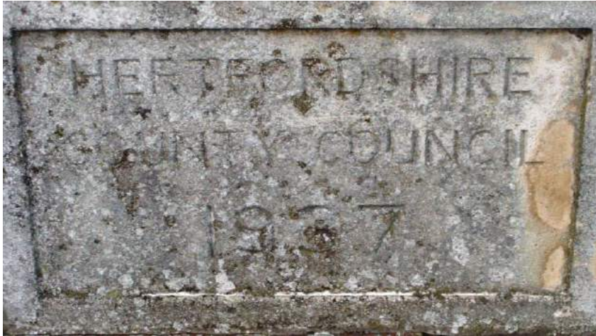
Picture 42. Plaque on bridge over River Rib needs re-inscribing to retain information for the future.
