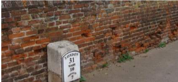
Picture 7. Repairs to spalled brickwork to St Peter's church may be eligible for grant assistance. Note the Milestone is also individually listed (the new metal plaque was attached in 2006).
