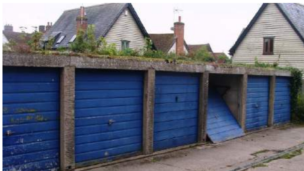
Picture 55. Poor quality lock up 'garaging' area that detracts. It is proposed to be removed from the Conservation Area. Despite this can any improvements be made. What is its future?
