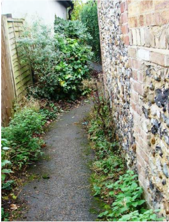
Picture 60. Removal of excess vegetation on footpath linking Pig's Nose and The Causeway would be advantageous.
